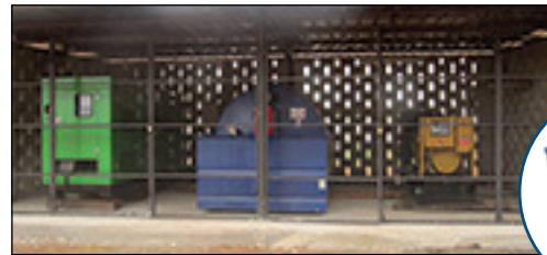
Diesel tanks - Generator sets
